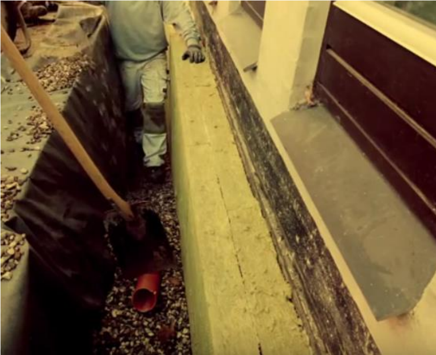
Figure 36. Foundation and footing insulation together with establishment of peripheral drainage around the building.
