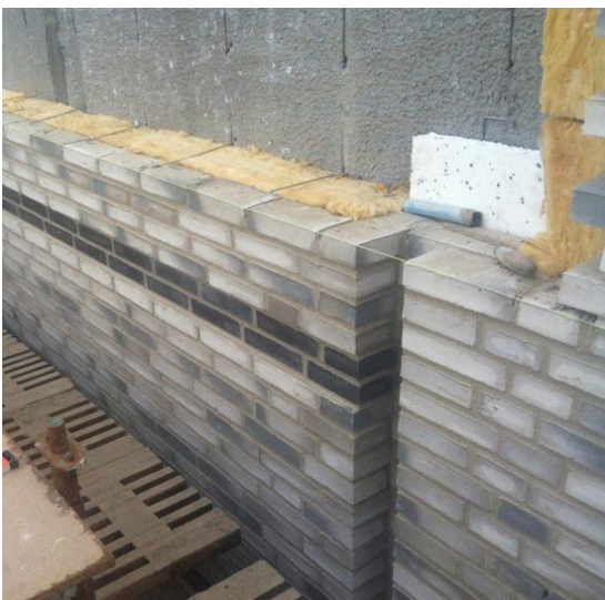
Figure 14. Demolition of external brick work, new thicker insulation and brick work- solution requires additional foundation.
