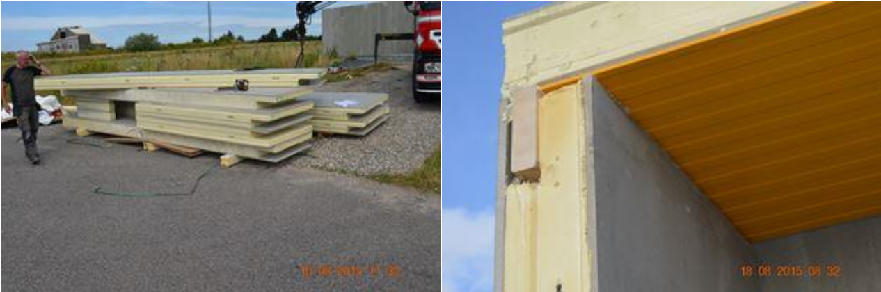
Figure 21. (Left) PUR panels delivered on the site, (right) panels assembly in the new house.
