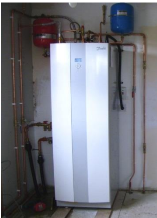
Figure 42. Heat pump with its connection pipes.
